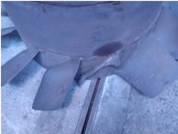
Analysis of the fracture edge reveals a typical fatigue crack.
